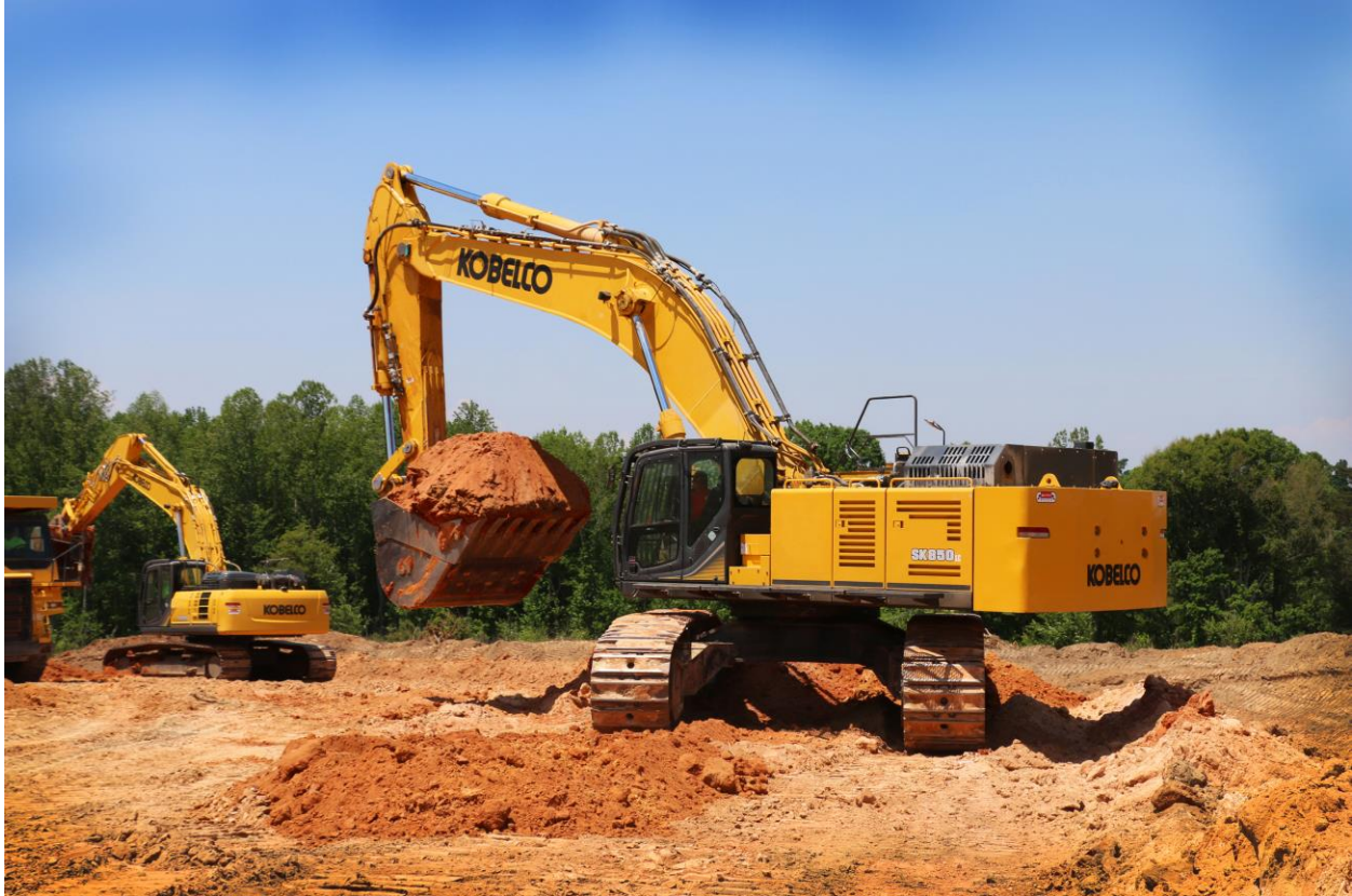
Photo Caption 3: KOBELCO excavators prepare the site for the company's new North American manufacturing facility.
