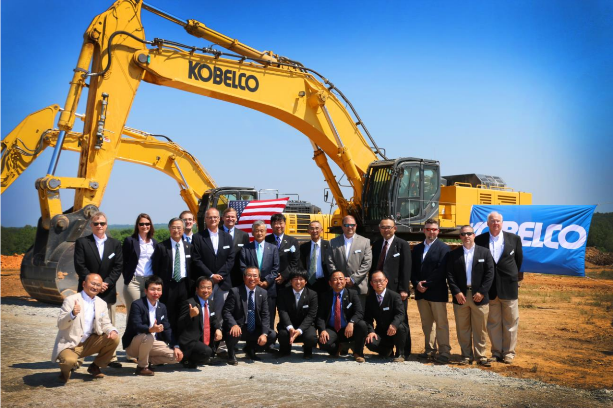
Photo Caption 2: The KOBELCO team breaks ground on their North American production facility in Spartanburg, SC.
