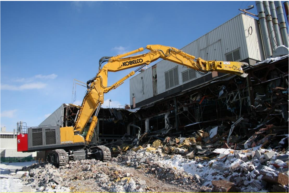
Photo Caption 2: The KOBELCO SK1000 working on site at the General Motors assembly plant in Oshawa, Ontario.
