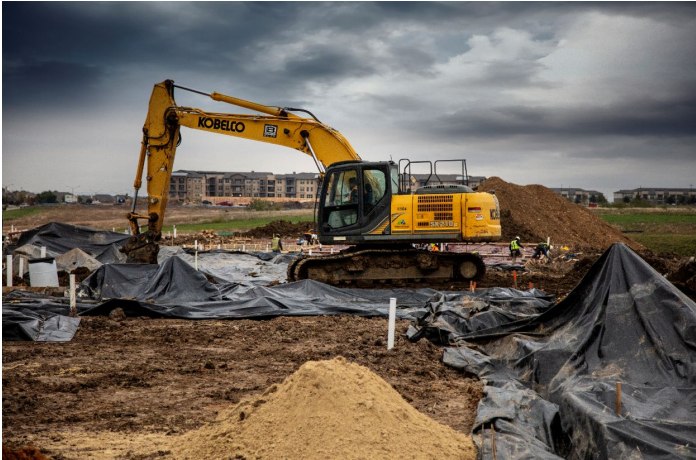
Photo Caption 3: The KOBELCO SK210LC on a Moss Utilities residential construction project in Texas.
